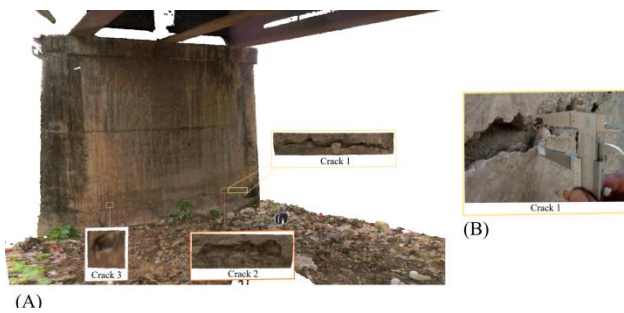
Figure 8. (A) Scanned cracks using TLS (B) Measurement of crack 1 using Vernier scale
